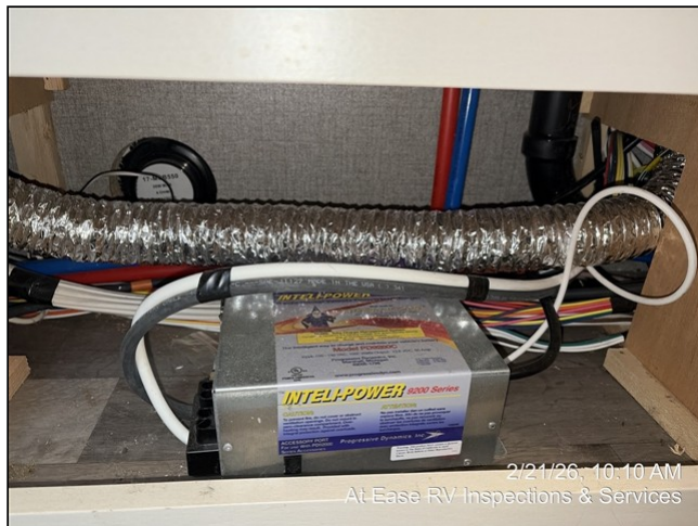
18.40 Item 1 (Picture) Converter/inverter
