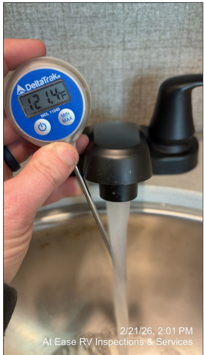
23.24 Item 2 (Picture) Hot water temp on electric
