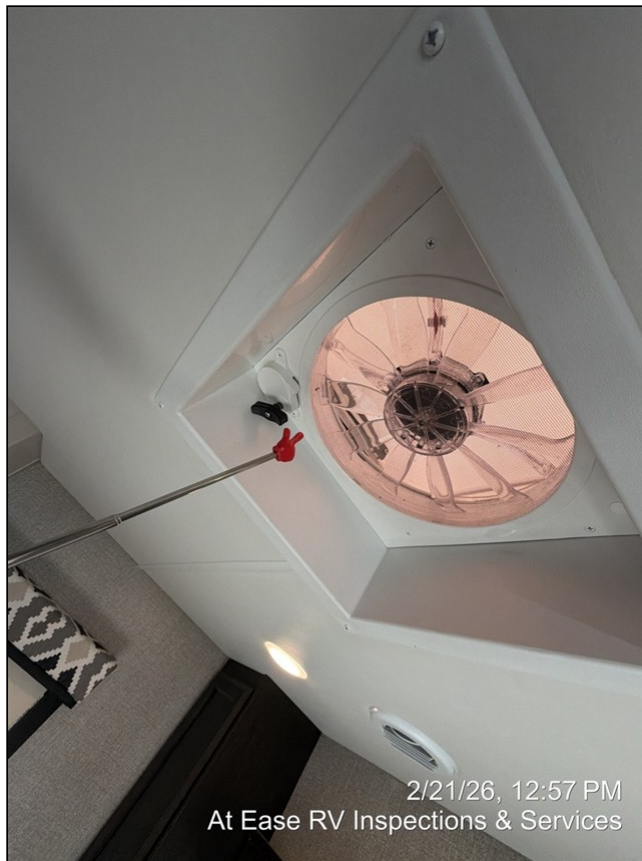
24.12 Item 1 (Picture) Vent in bedroom
