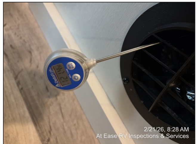
21.7 Item 2 (Picture) Output temp near bathroom sink
