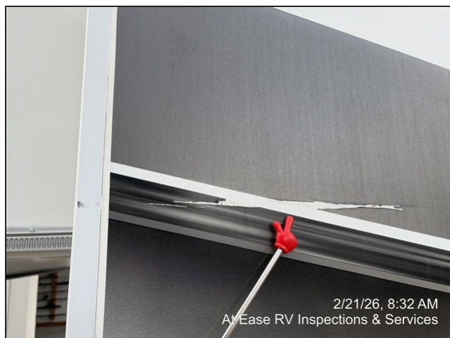
6.0.B Item 1 (Picture) Surface scratch at back
