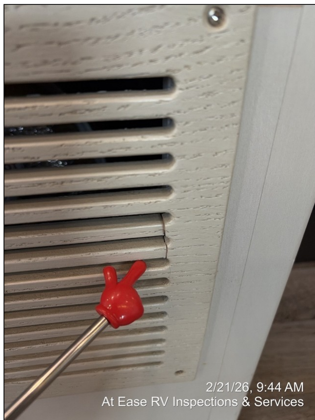
24.24 Item 1 (Picture) Water heater access panel
