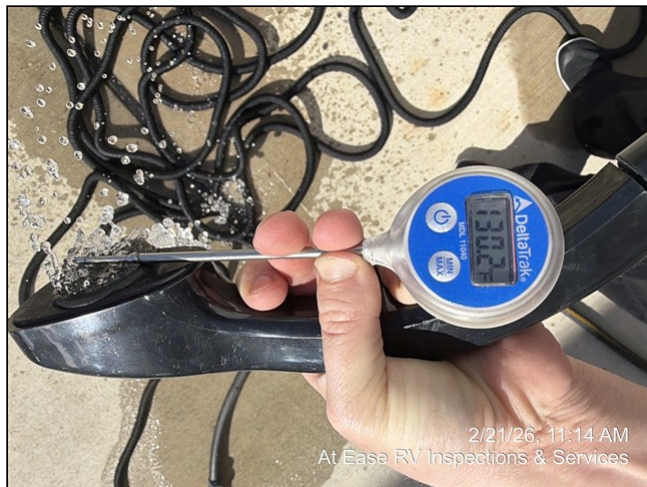
19.4 Item 1 (Picture) Hot water temp
