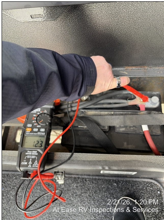
18.30 Item 1 (Picture) Battery without shore power
