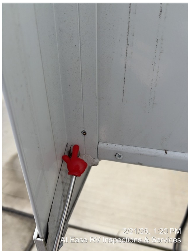
12.5.B Item 1 (Picture) Screw head broken off
