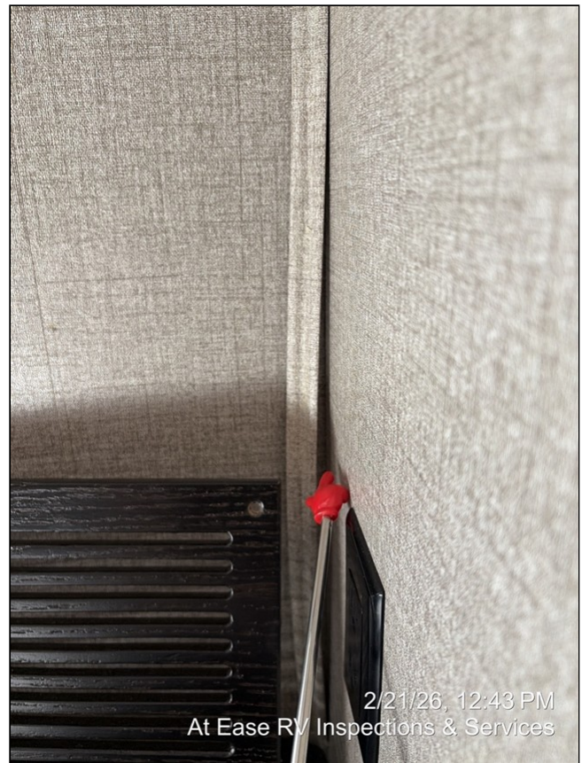
24.28 Item 2 (Picture) Trim in bedroom
