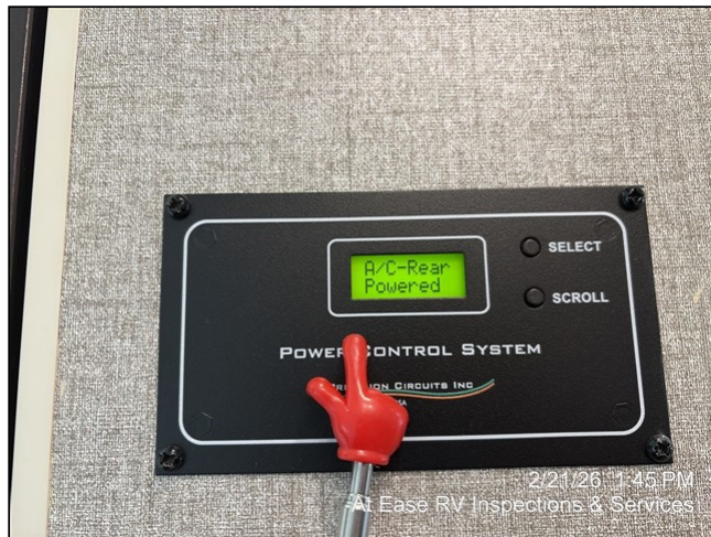
18.18 Item 1 (Picture) Power control panel
