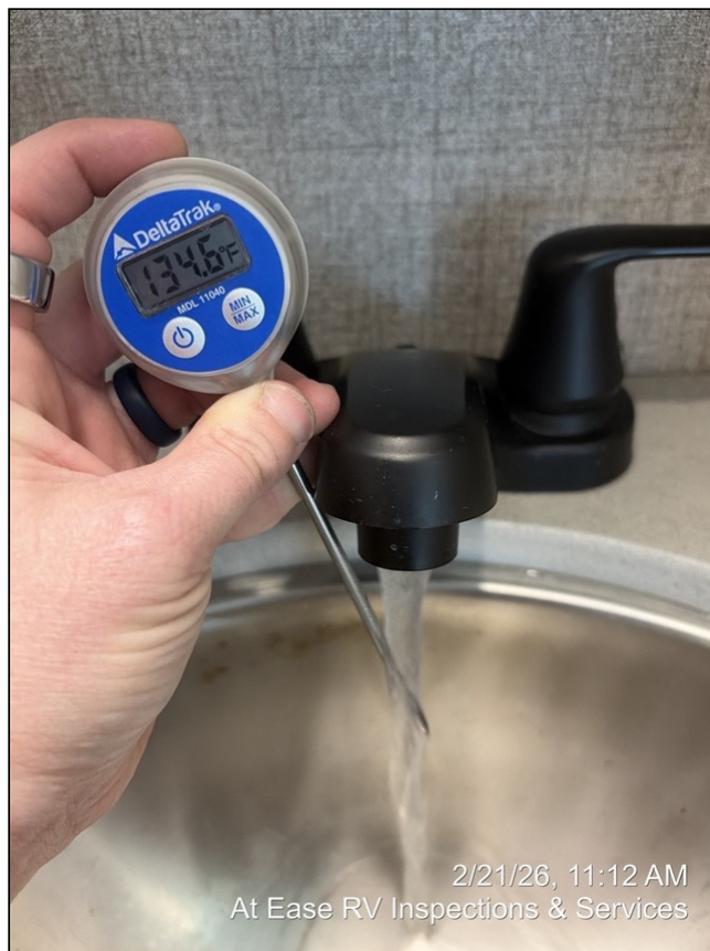
23.24 Item 1 (Picture) Hot water temp on gas
