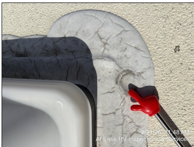
8.6 Item 2 (Picture) Popped bubble
