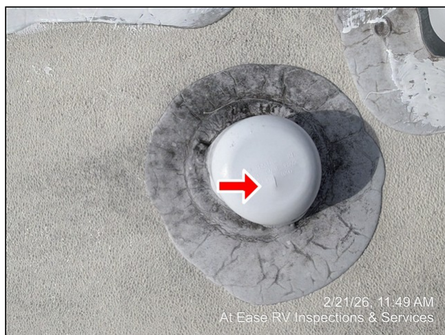
8.8 Item 1 (Picture) Plumbing vent cap
