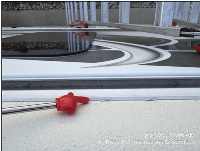
8.2 Item 1 (Picture) Cracks in sealant
