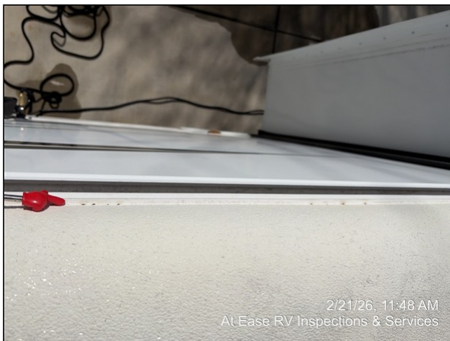
8.4 Item 1 (Picture) Gaps in sealant on trim rail
