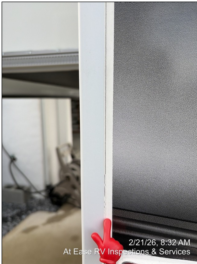
6.2.B Item 1 (Picture) Sealant along the rear wall joint
