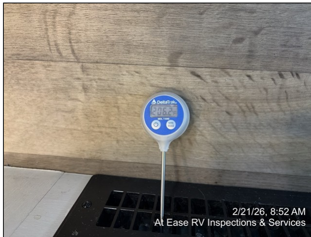
21.7 Item 3 (Picture) 2nd kitchen vent output temp
