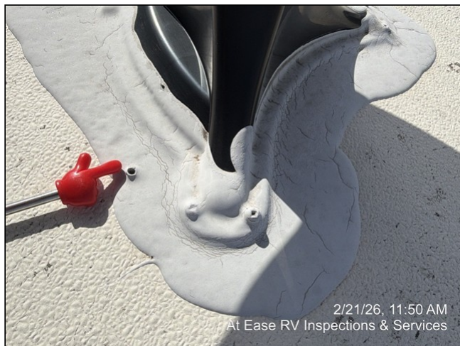
8.13 Item 1 (Picture) Popped bubble in sealant
