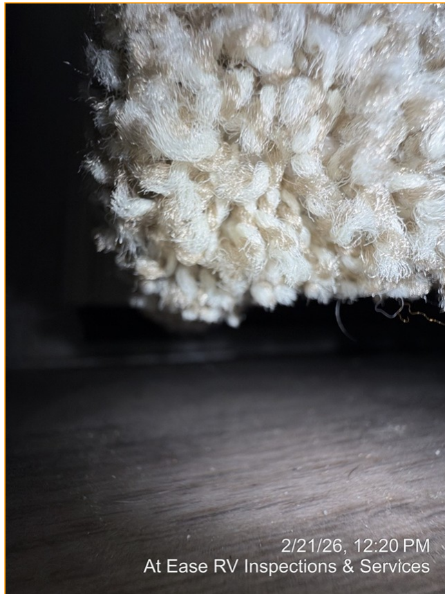
24.51 Item 5 (Picture) Under slideout corner
